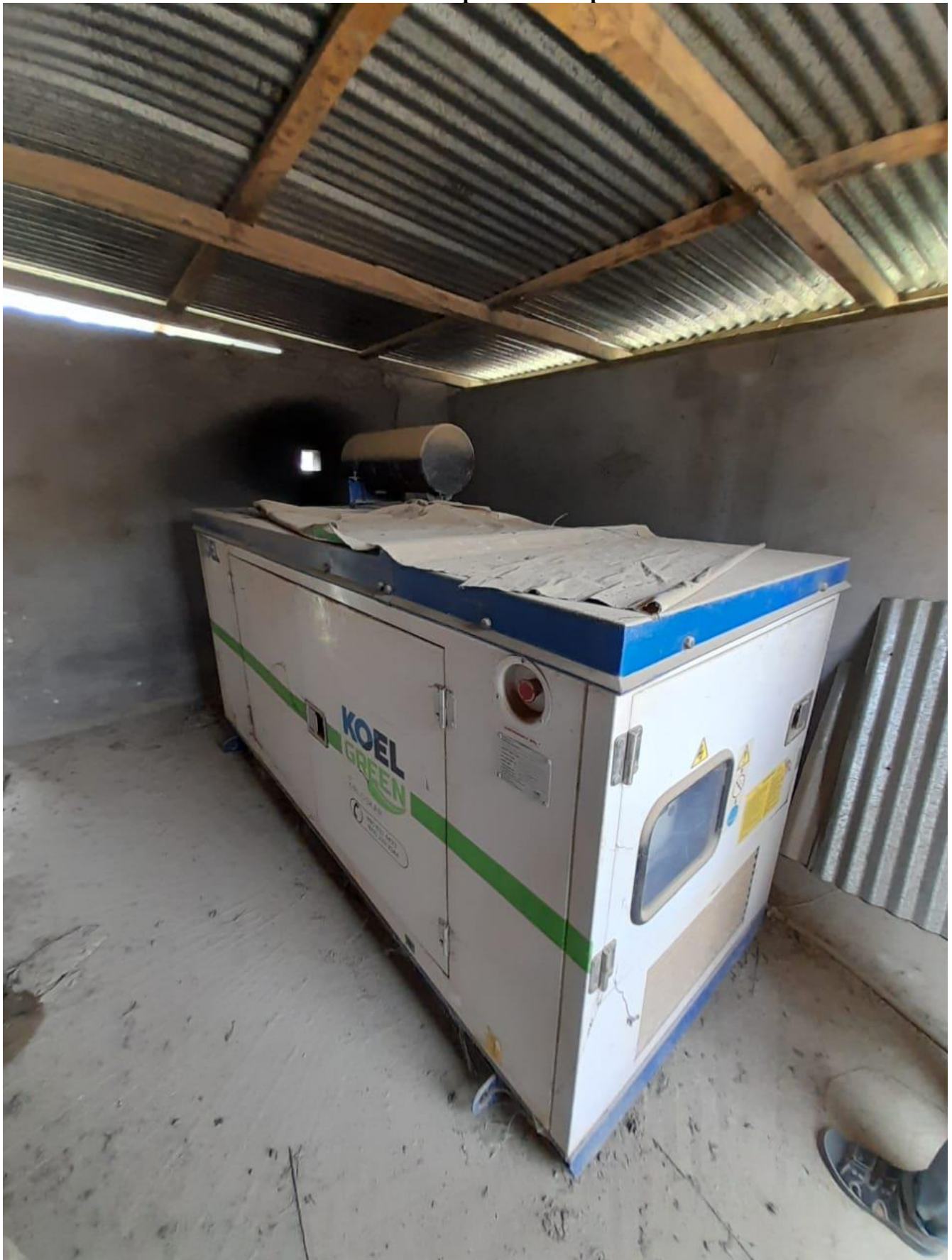
Generator for power Backup-1
