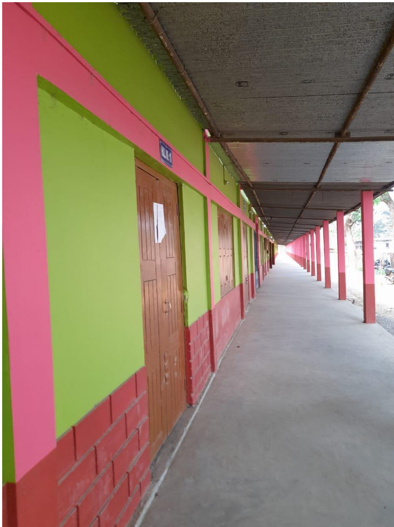
Block-D Science class room, Central Library, Auditorium hall, Psychological Laboratory.
