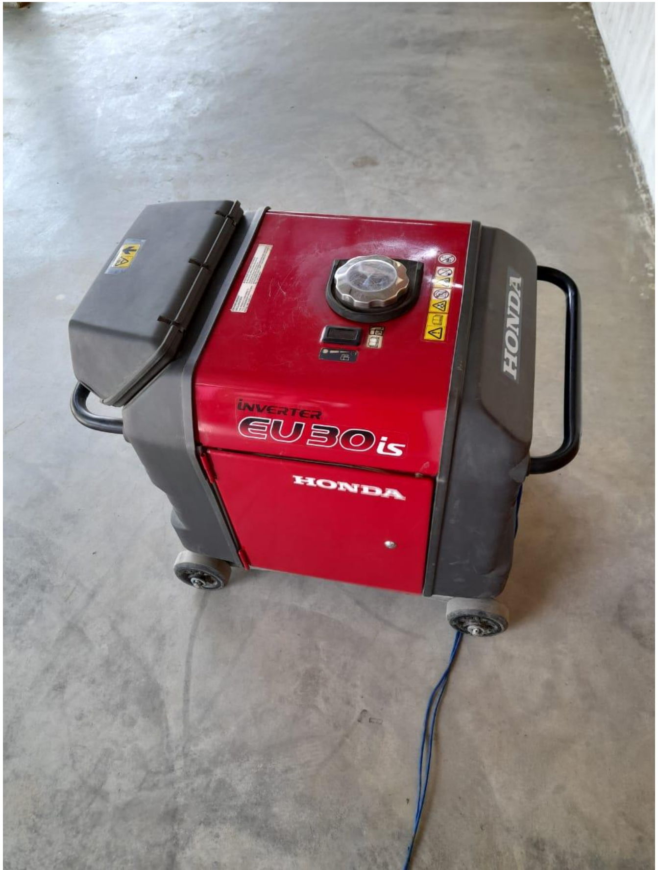
Generator for power Backup-2
